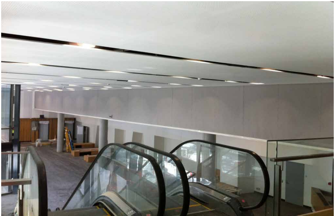
| The Supercoil long span smoke curtain installed at the Brisbane Convention & Entertainment Centre
